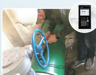
Cooling Water Measurement
